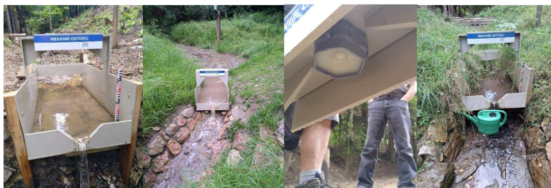
Figure 21 : Water flow measurement stations with online data transmission
